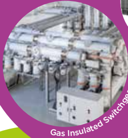
Gas Insulated Switchgear
